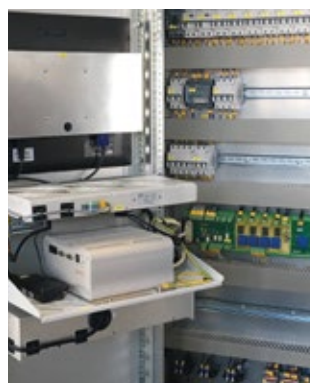
Cabinet with minimum amount of hardware and standard components.
